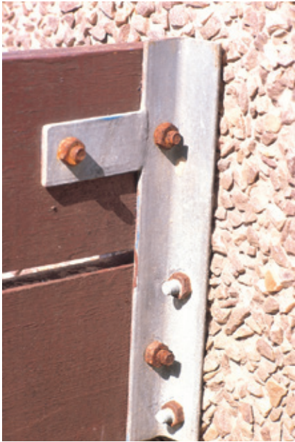
Figure 1: An assortment of zinc coated bolts showing the importance of coating thickness in a particular environment.
