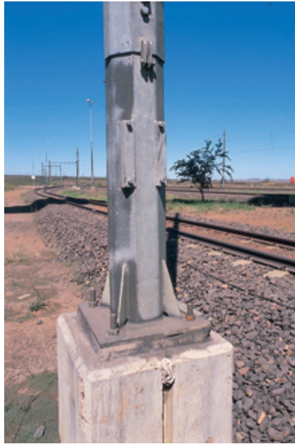
Figure 2 (above) and Figure 3 (above right): Corrosion protection of holding down bolts should be equal to that provided for main structures.
